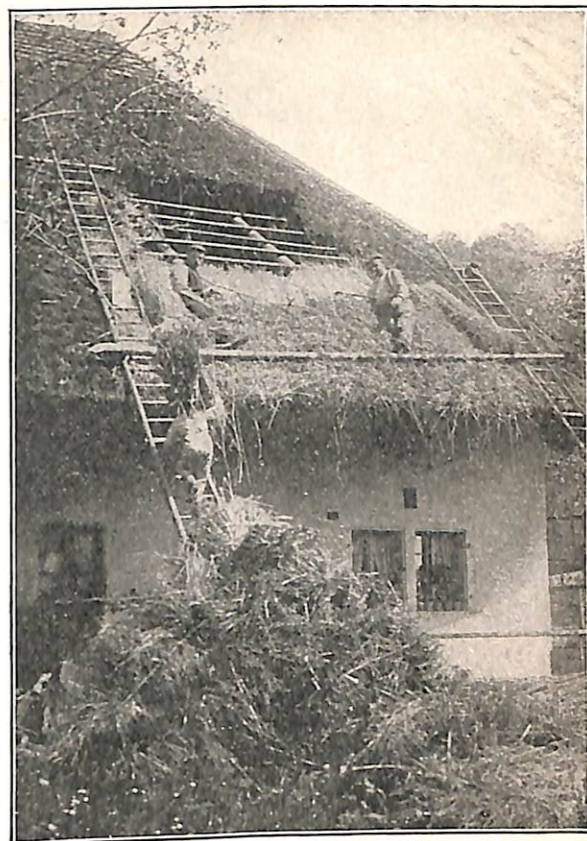
Fig. A. This farmhouse in Switzerland has a thatched roof. The workmen are repairing the roof with straw.
